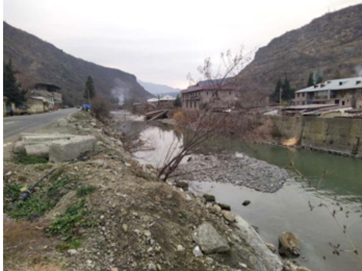
Image 4. Destroyed road at Karkop
