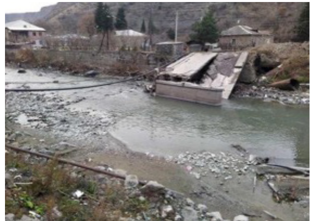
Image 15. Destroyed bridge in Karkop village
