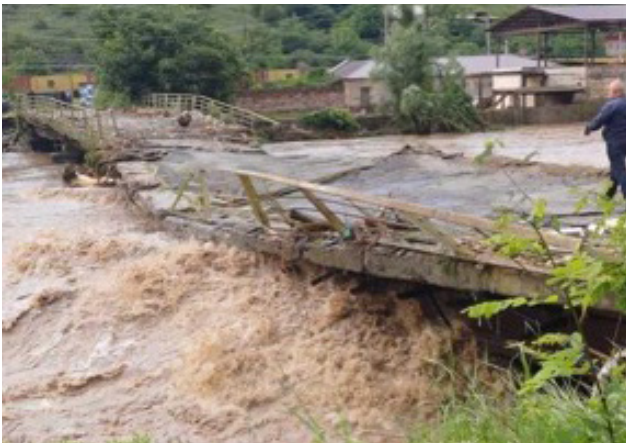
Image 16. Ayrum bridge during the flood
