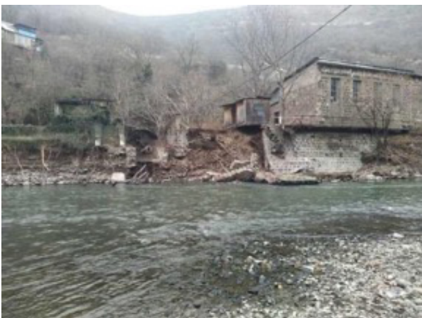
Image 20. Debed river with destroyed bank protection works at Sanahin
