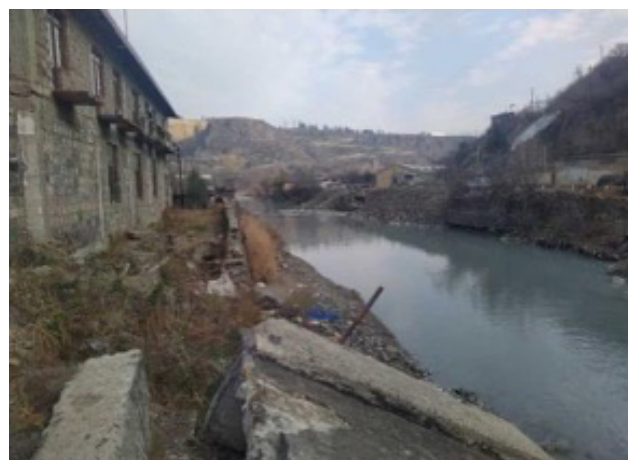
Image 21. Destroyed bank protection works at the right side of Debed river at Karkop
