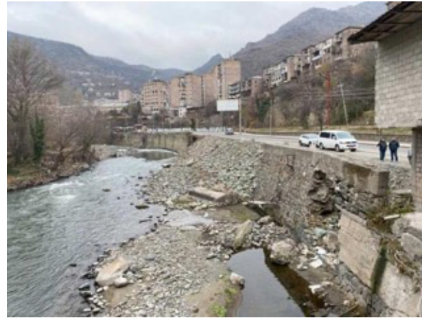
Image 26. Collapse of the protection wall downstream of the dam
