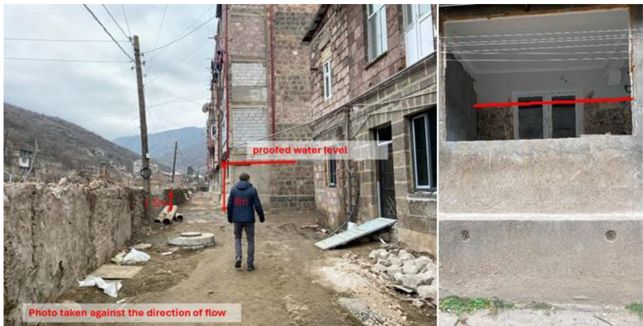
Image 33. Height of protection wall and damages / proofed water level compared to path on the west bank of Debed river in Sanahin station.
