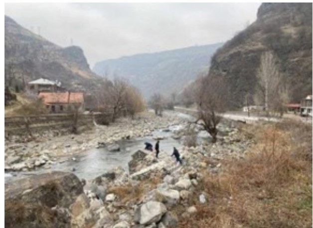
Image 19. Collapsed bank protection works below the confluence of Pambak and Dzoraget rivers
