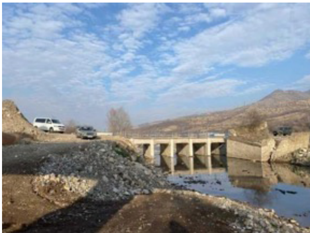
Image 18. Undercut lateral protection works
