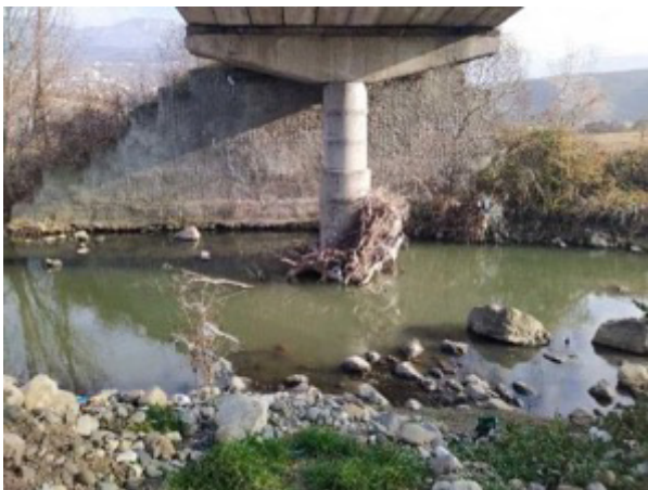
Image 10. Khashtarak bridge with undercut sidewall
