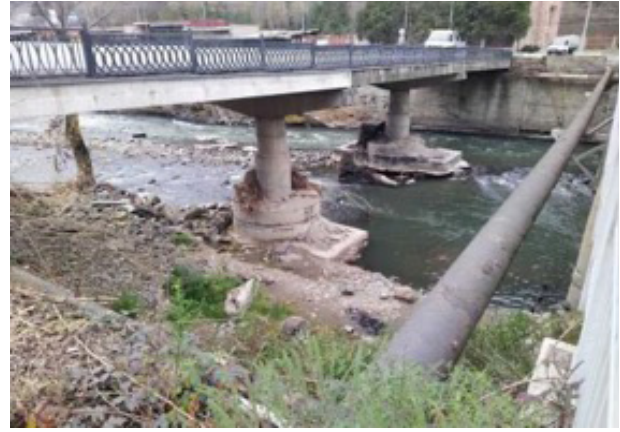
Image 13. Undercut piers of bridge in Alaverdi
