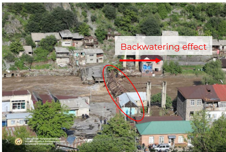
Image 34. Backwatering effect through damaged bridge in sanahin station:
