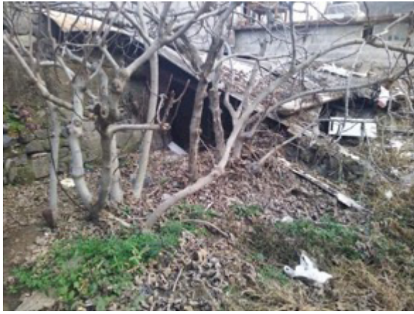
Image 6. Wall with hole were water entered the village of Karkop
